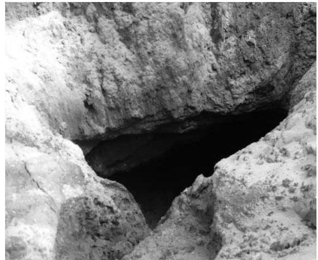
Fig. 1. Sinkhole subsidence in an area of shallow mining works at the JK mine in Jaworzno (photo: R. Jendruś).
