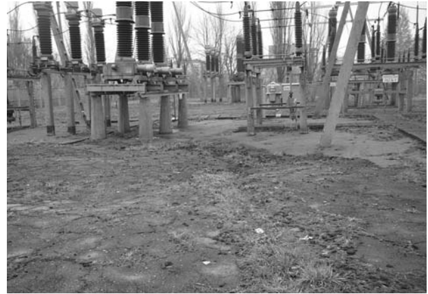
Fig. 4. Sinkholes and tilted poles at the Julian Power Distribution Centre (photo: R. Jendruś).
