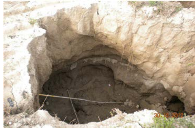
Figure 2. Signs of piping along the fissure. Soil erosion caused by water beneath the surface of the ground creating an underground tunnel.
